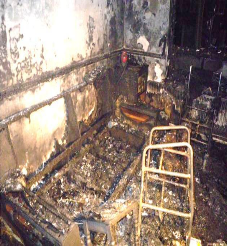
Fire damage in living room
